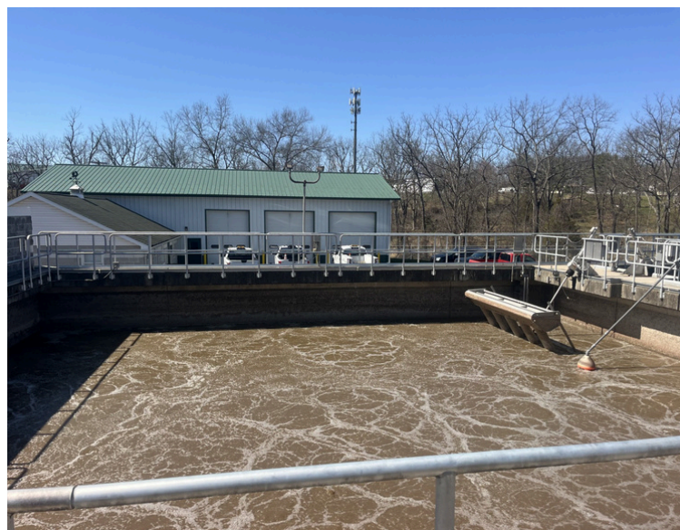
This is an SBR basin. Raw sewage is pumped in here and treated via aeration, settling, and decanting. Clear water is skimmed off the top and treated, solids move to the SBR tank. It's a poop stew!
